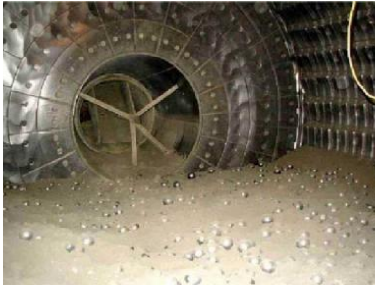
Fig. 2: Ball mill for cement grinding (Source: Chr. Pfeiffer Beckum)
